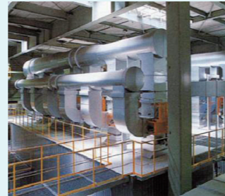
Equipment eliminates pollutants in factory exhaust gas.
