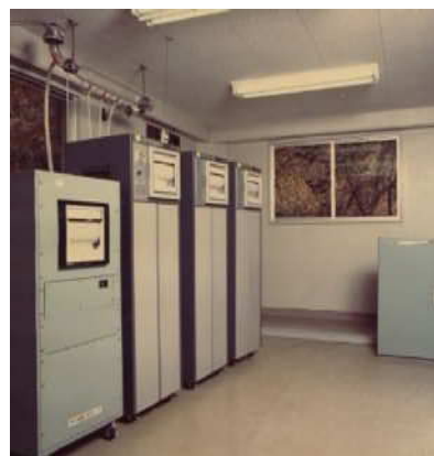
Air monitoring equipment
