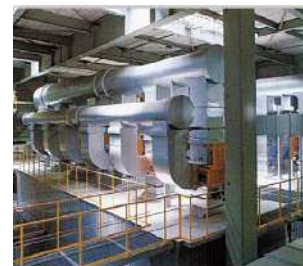
Smoke scrubbing equipment
