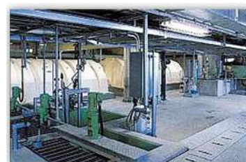
Wastewater treatment equipment
