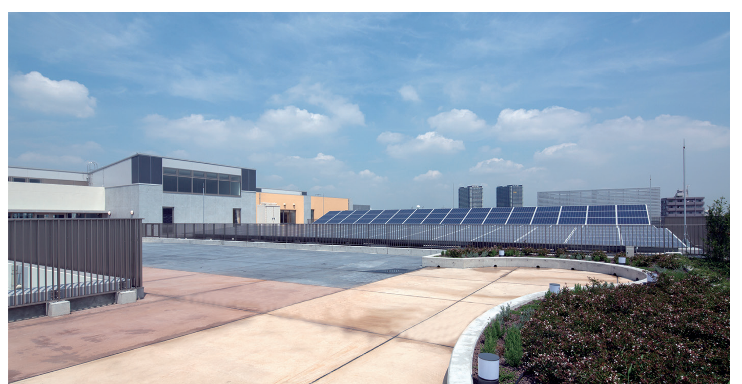
Solar panels on school rooftops
