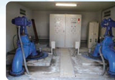
Ikuta Bored Well Ground water is pumped up from 6 bored wells (shallow wells) in Tama Ward.
