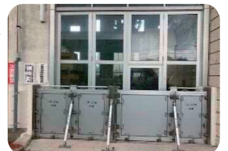
Waterproofing of facilities (watertight panels)
