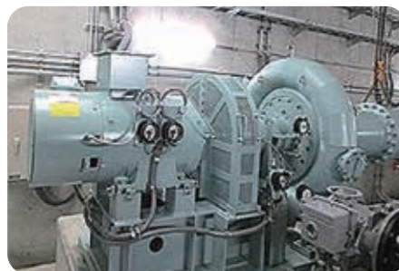
Hirama Power Plant Facility
