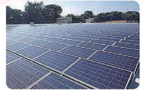
Ikuta Distribution Reservoir Solar Power System
