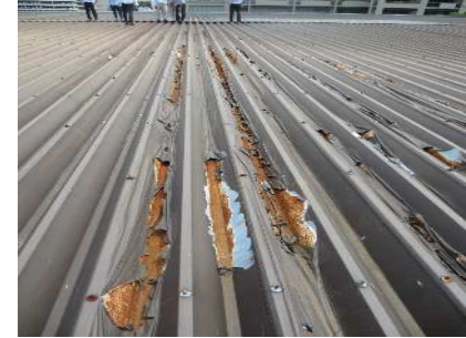
折板塗装はく離
