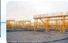
リーファ電源 Power points for a refrigerated container
