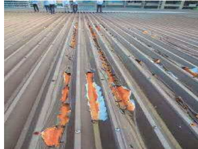
折板塗装はく離
