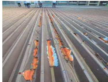
折板塗装はく離
